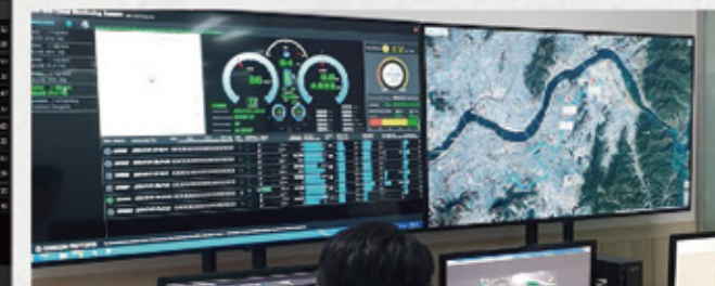
Integrated Control Room Big Data Management
